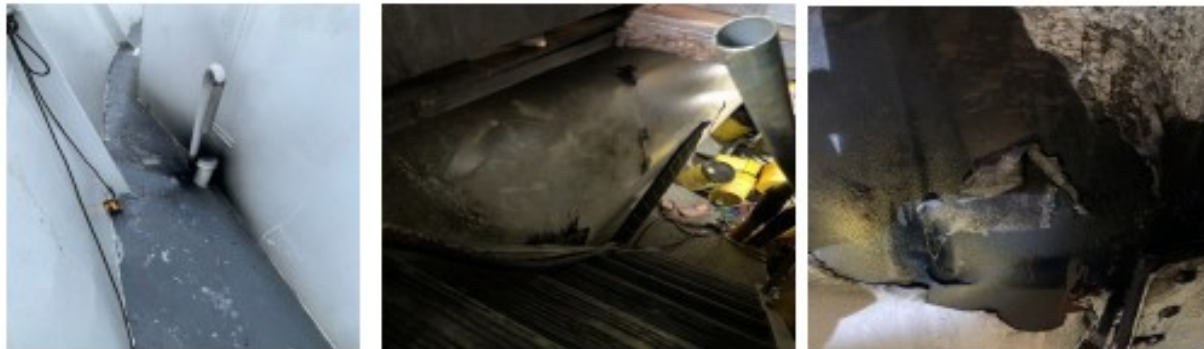
Figure 1-Left: Fuel tank vent pipe (soot residual from explosion), Center: Bulkhead between fuel tank and engine room (ballooned/explosion), Right: Ruptured bulkhead (fractured from explosion).
