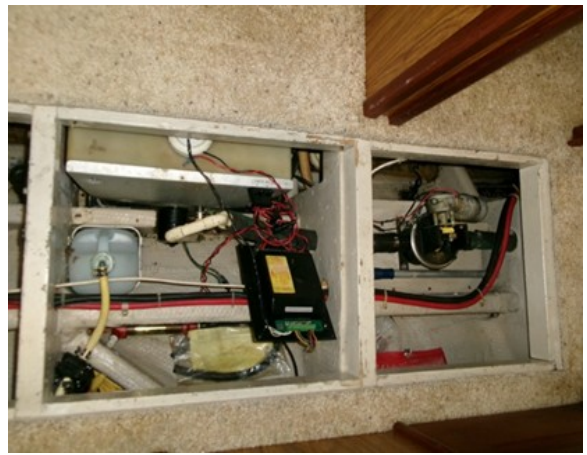
Forward floorboard access old system
